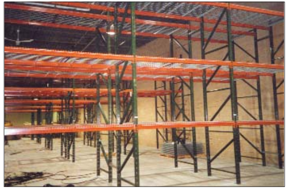
Pallet Rack installation by Ted Thorsen LLC. Base Pads are being lagged to the floor and decking is being positioned.
